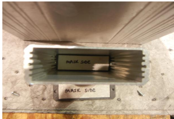
Post-Dust/Water Intrusion Inspection - 8/6/2011
