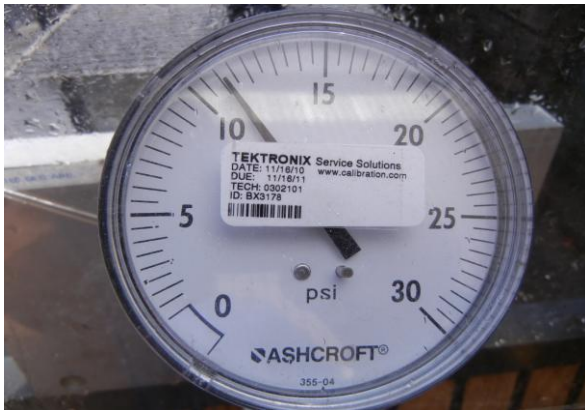
Water Pressure ( Typical) - 8/4/2011
